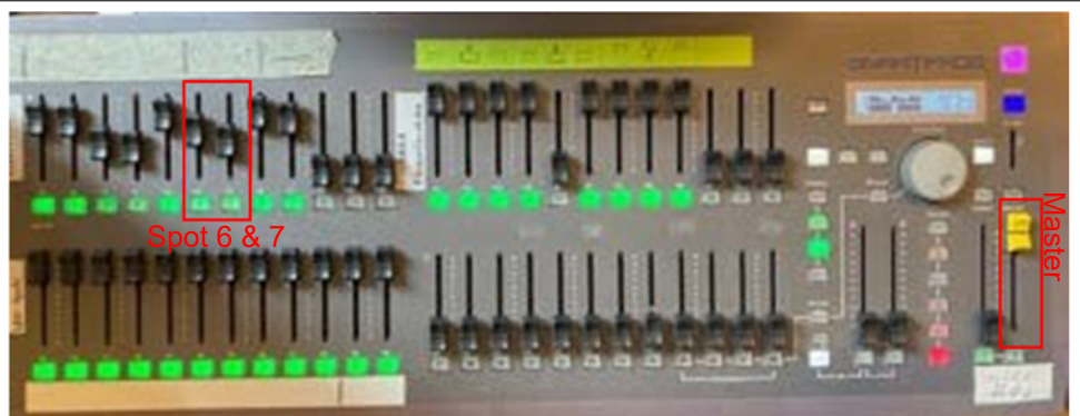
Picture 10: Light controller
